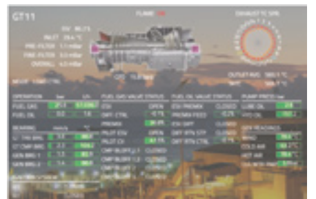
Gas turbines monitoring
